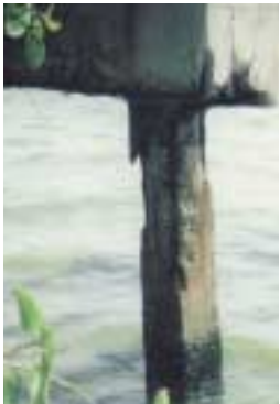
Corroding concrete piling
